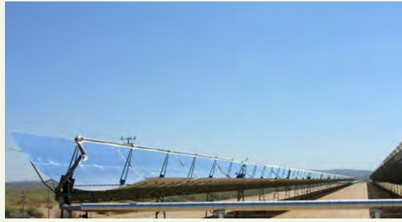
Figure 25.44 Parabolic trough collectors are used to generate electricity in southern California. (credit: kjkolb, Wikimedia Commons)
