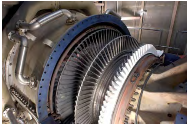
Figure 23.24 Steam turbine/generator. The steam produced by burning coal impacts the turbine blades, turning the shaft which is connected to the generator. (credit: Nabonaco, Wikimedia Commons)
